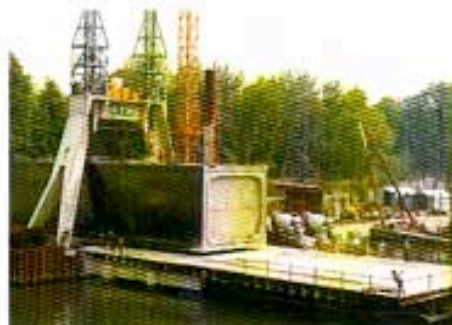
A section is laid under the Seine in Paris. Built by GTM Entrepouse for the RATP Metro system.
